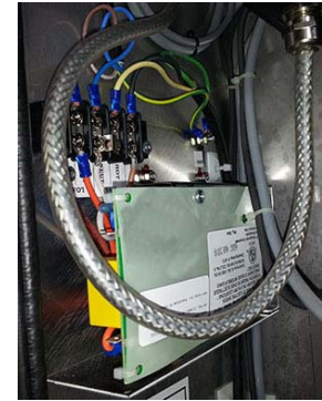
Installed in Machinery
