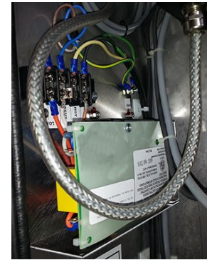
Installed in Machinery
