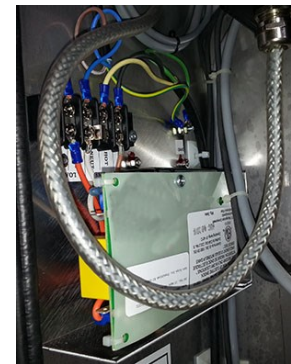
Installed in Machinery
